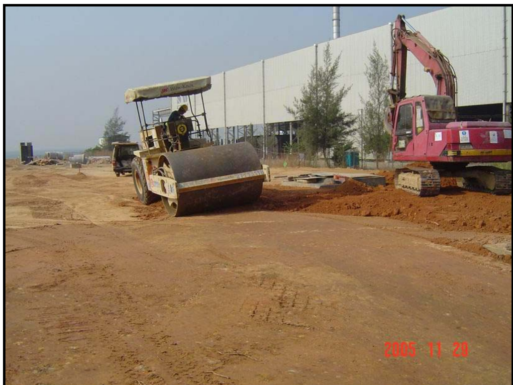
Figure 8 General condition of access road to PAFF Construction Site (Photo: Leighton Contractors (Asia) Limited, November 2005)
