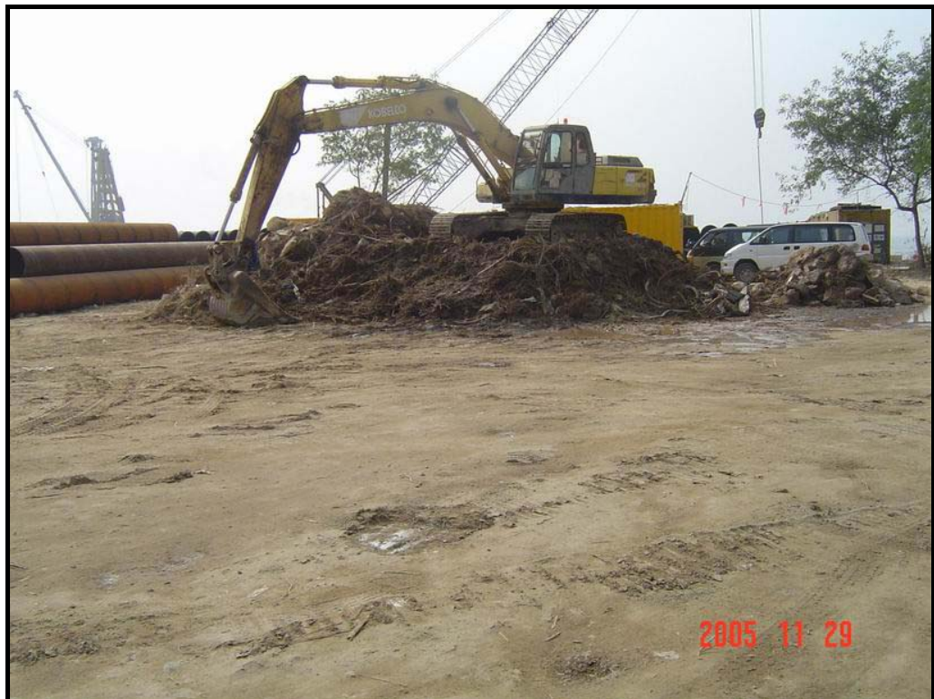
Figure 6 Small stockpile doused with water at PAFF Construction Site (Photo: Leighton Contractors (Asia) Limited, November 2005)
