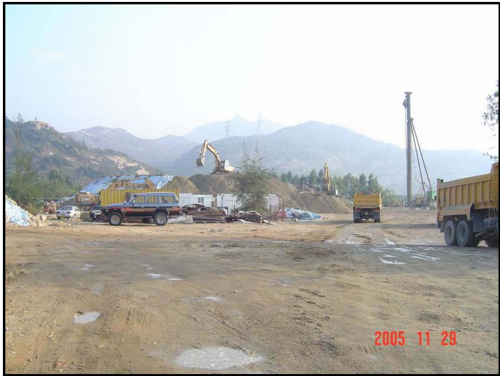
Figure 5 Sand surcharge partially covered with tarpaulin at PAFF Construction Site (Photo: Leighton Contractors (Asia) Limited, November 2005)
