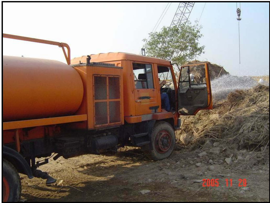
Figure 3 Water Truck dousing stockpile at PAFF Construction Site (Photo: Leighton Contractors (Asia) Limited, November 2005)
